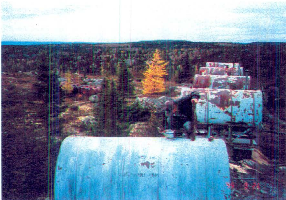
Site 333. Checking diesel reservoirs for residue.
